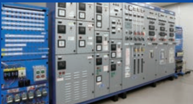
Low-voltage switchboard and Starter Panel simulators
