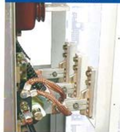
Closing Earthing Switch
