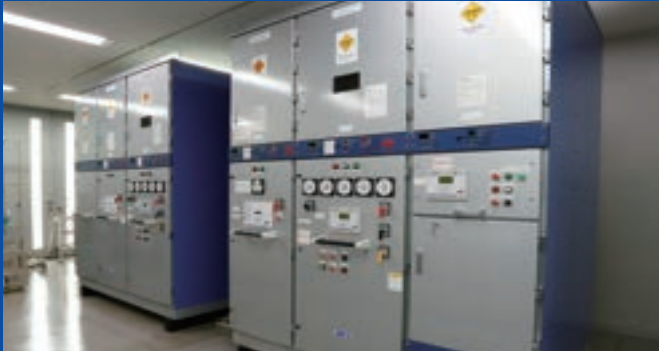
High Voltage Switchboard Simulator
